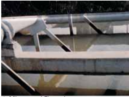
1. Mixers and Flocculators
