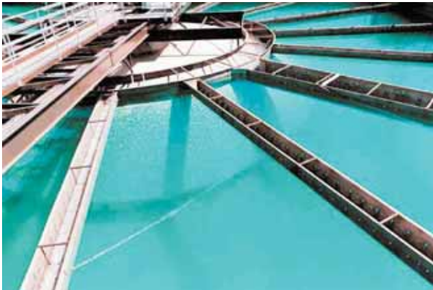
HRC Mechanism used in municipal softening
